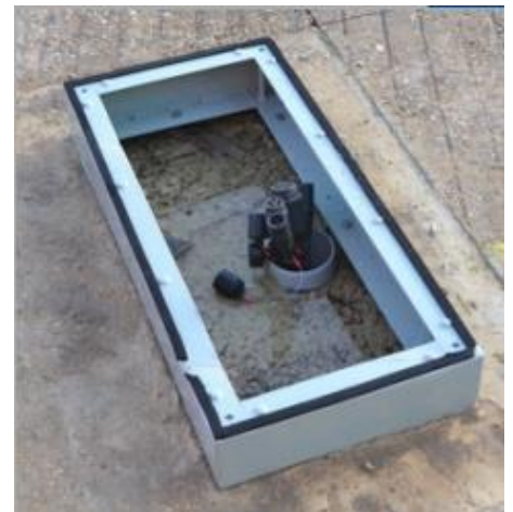
Figure 5 - Cabinet base (cassette) after breakaway
