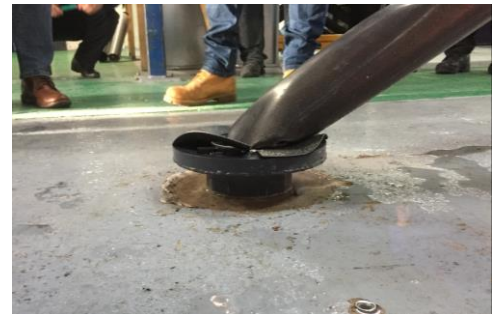
Figure 1 - Damaged Pole in Atlas Socket
