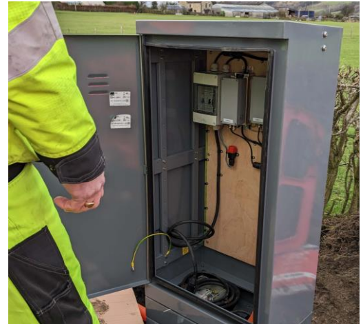
Figure 13 – On-site installation of a Passively Safe Cabinet with the impact sensor installed on the top half of the backboard.
