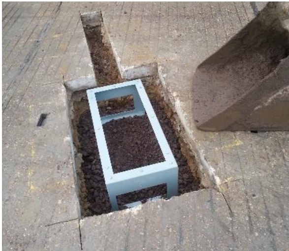
Figure 1 - Plinth is placed in a hole of adequate size and the feet are secured using gravel/dry mix concrete.
