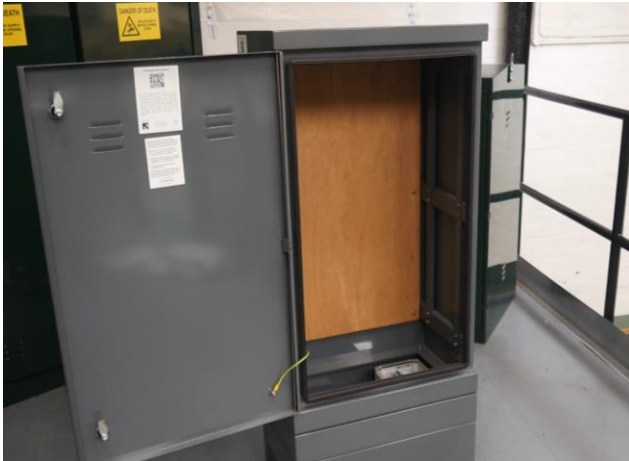
Figure 9 - Cabinet placed on top of the cassette-plinth with the shear-bolt ends visible inside the cabinet.
